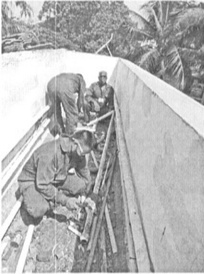
Plumbers & Welders are replacing the rusted and leaking water lines of Sagaresh Hostel.
